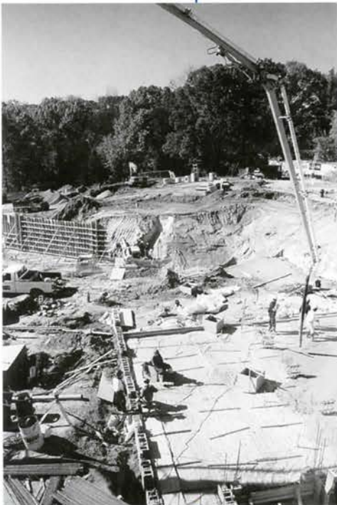
Construction crews pour the concrete foundation of The Engelhard Performing Arts Center, Fall 1999
